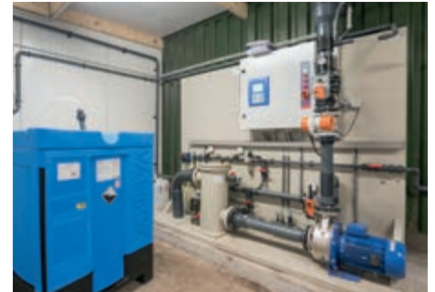
Technical room with acid container
