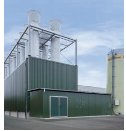
Exhaust air tower with integrated Pollo-M
