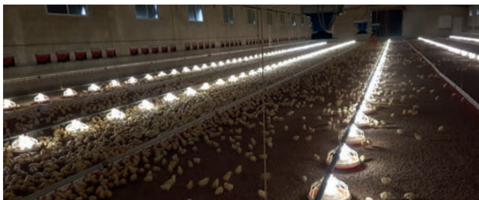
Use of FlexLED glo in a broiler house
