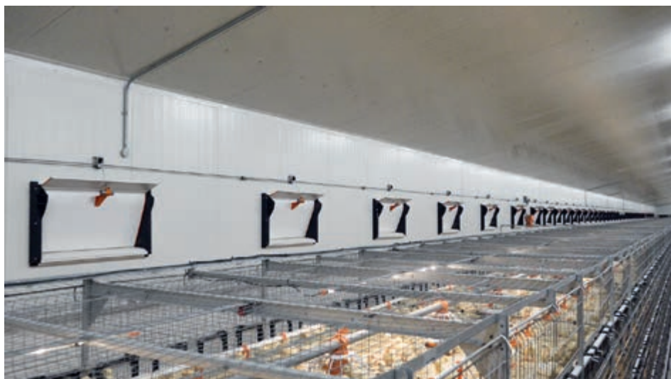
AviMax transit: fresh air supply through the CL Flex flange inlet
